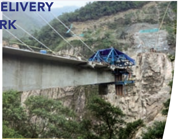
Some works being currently constructed on a PPP Project in Colombia in a motorway connecting the cities of Bogotá and Villavicencio. The concessionaire of the project is Coviandes. Photo's by Felipe Castro Arenas.
